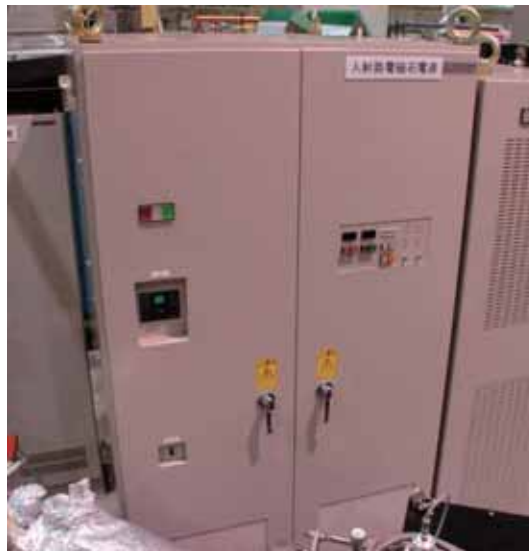
Fig. 2. New Magnet Power Supply for Bending Magnets on Beam Transport Line
